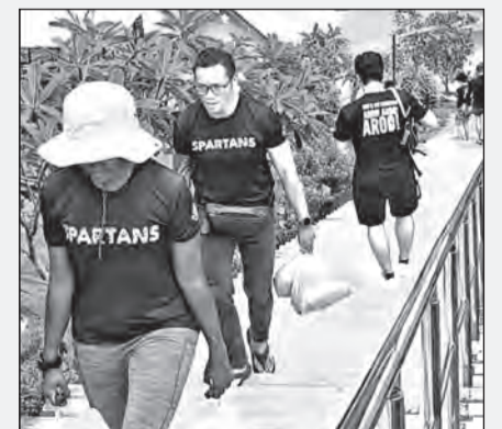
Dedicated volunteers transporting sand and cement to the front of Mt Hosanna Chapel.
